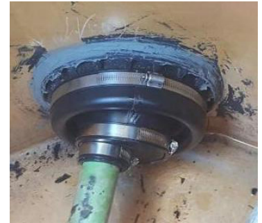
Example of Blueline Large KFD Repaired
