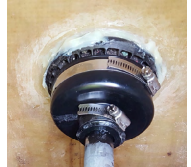
Example of BlueLine Small KFD Repaired
