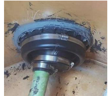
Example of Blueline Large KFD Repaired
