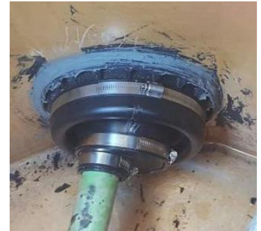
Example of Blueline Large KFD Repaired
