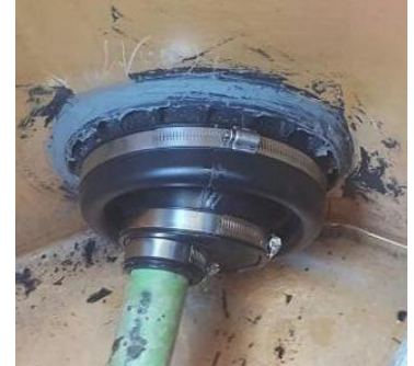
Example of Blueline Large KFD Repaired
