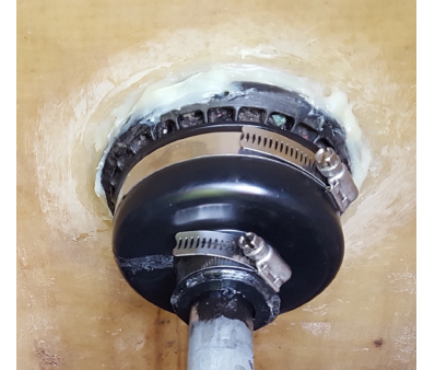
Example of Blueline Small KFD Repaired
