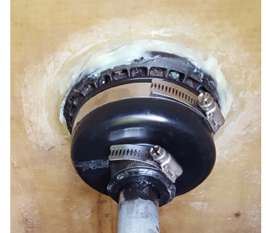
Example of Blueline Small KFD Repaired
