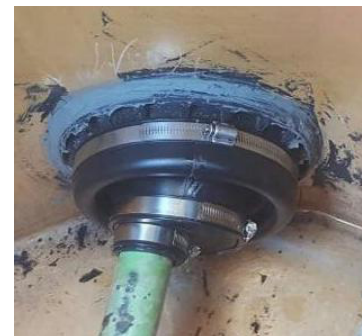
Example of Blueline Large KFD Repaired
